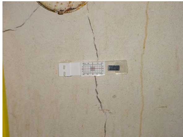
Avongard Monitor to Measure Crack Movement
